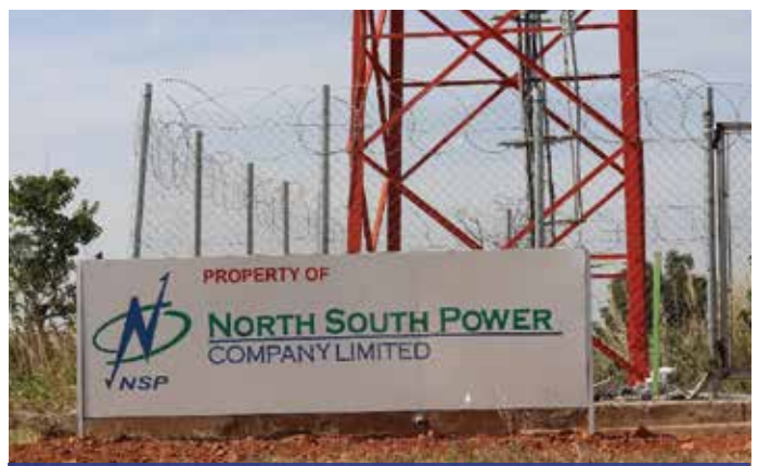
NSP COMMUNICATION MAST (FRONT VIEW)
